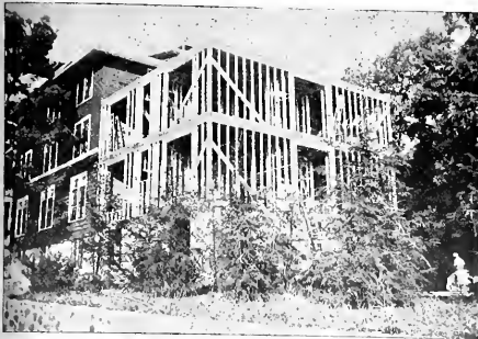
The new addition to the Girls' Dormitory will add twenty-eight rooms to the building. This picture was taken a short time ago and much has been added since, because of such rapid progress in the construction.
